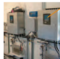
Field remote terminal.
