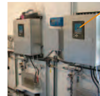
Field remote terminal.
