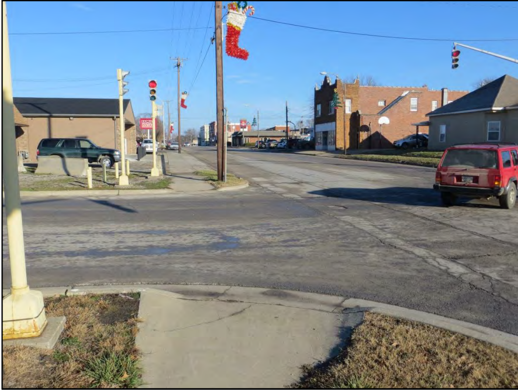
Figure 6 - Lack of Pavement Markings from Southwest Corner Looking North (6th St. & W. Pacific Ave.)
