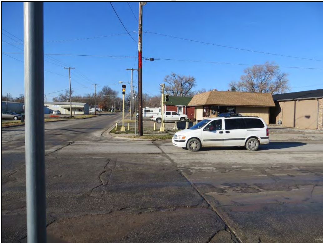
Figure 7 - Lack of Pavement Markings from Northeast Corner Looking West (6th St. & W. Pacific Ave.)
