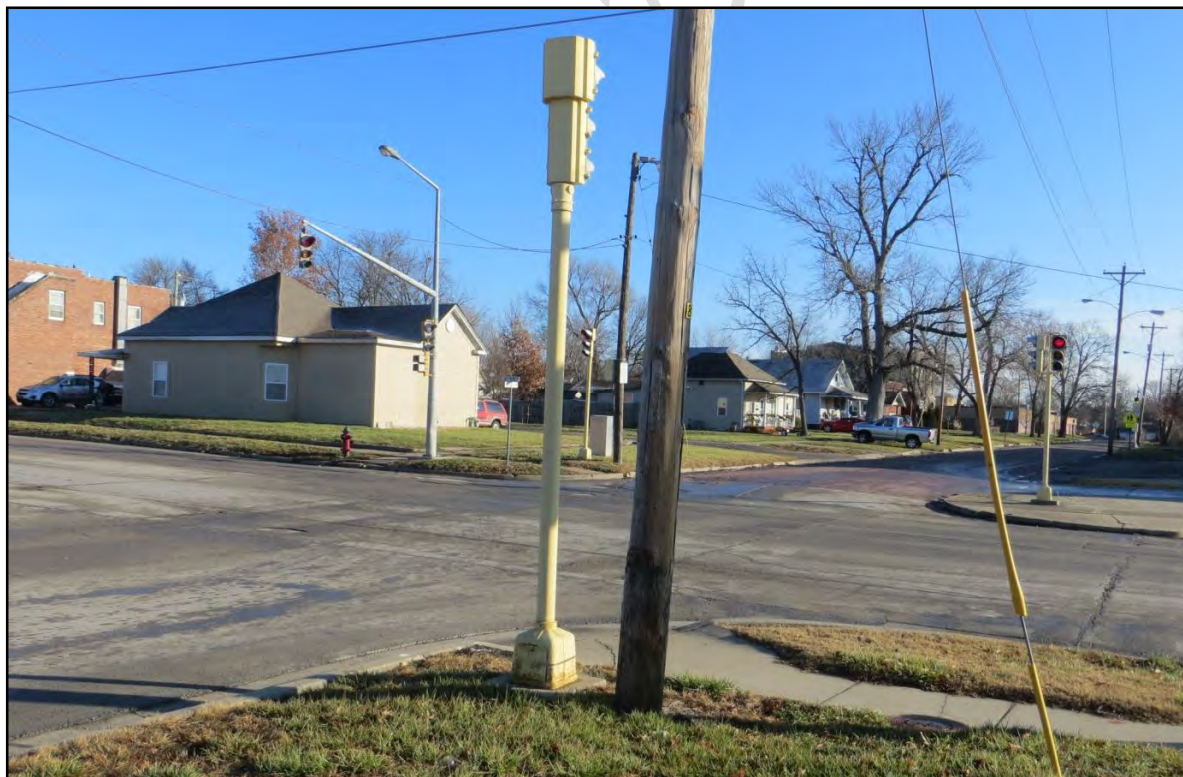
Figure 2 – Eastbound and Westbound Signals Mounted on Poles; Photo taken on the South West Corner (6th St. & W. Pacific Ave.)
