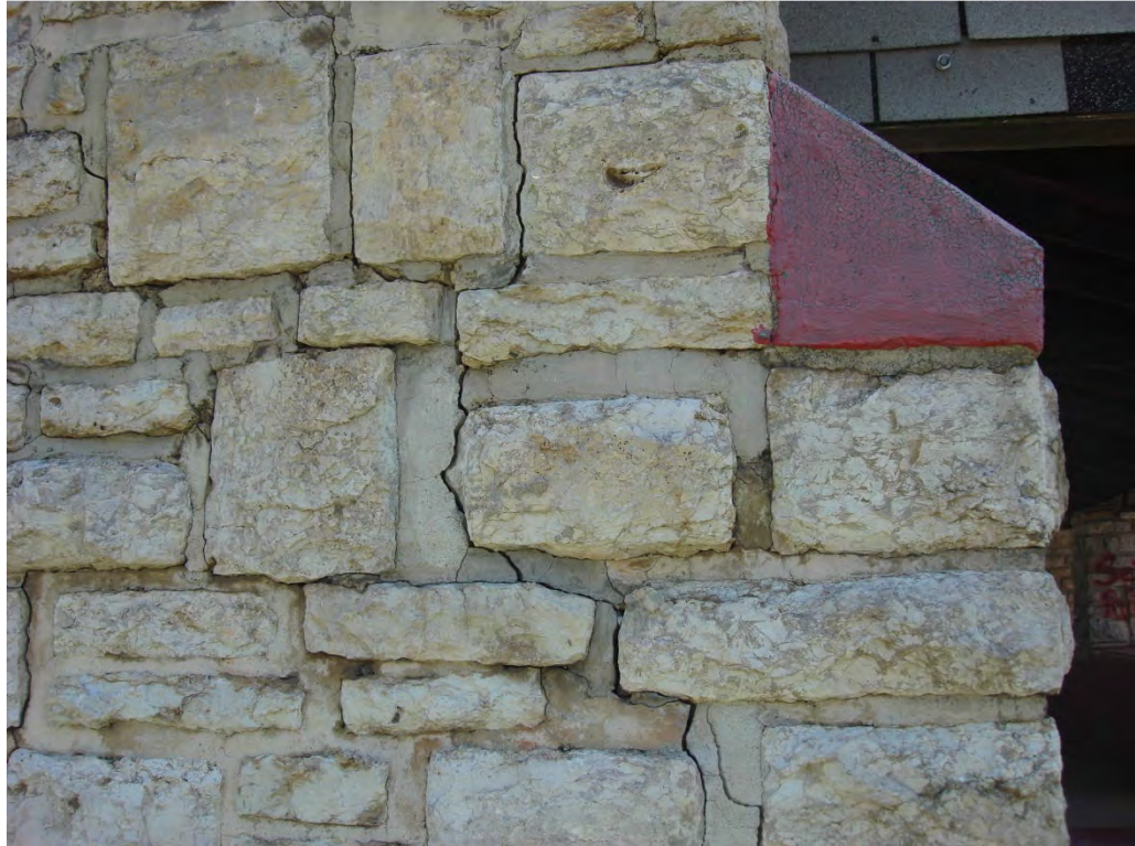
Typical cracks along mortar lines in chimneys
