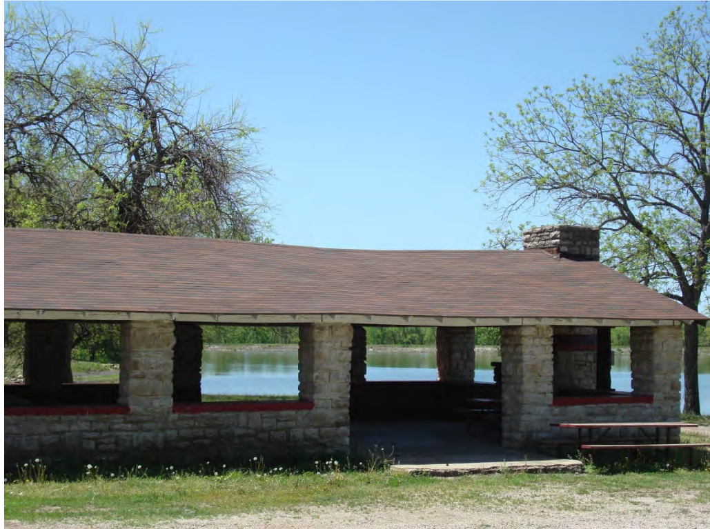
Sag in roof line ridge
