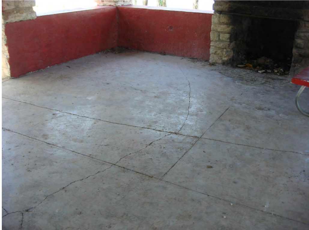
Charred fire place
