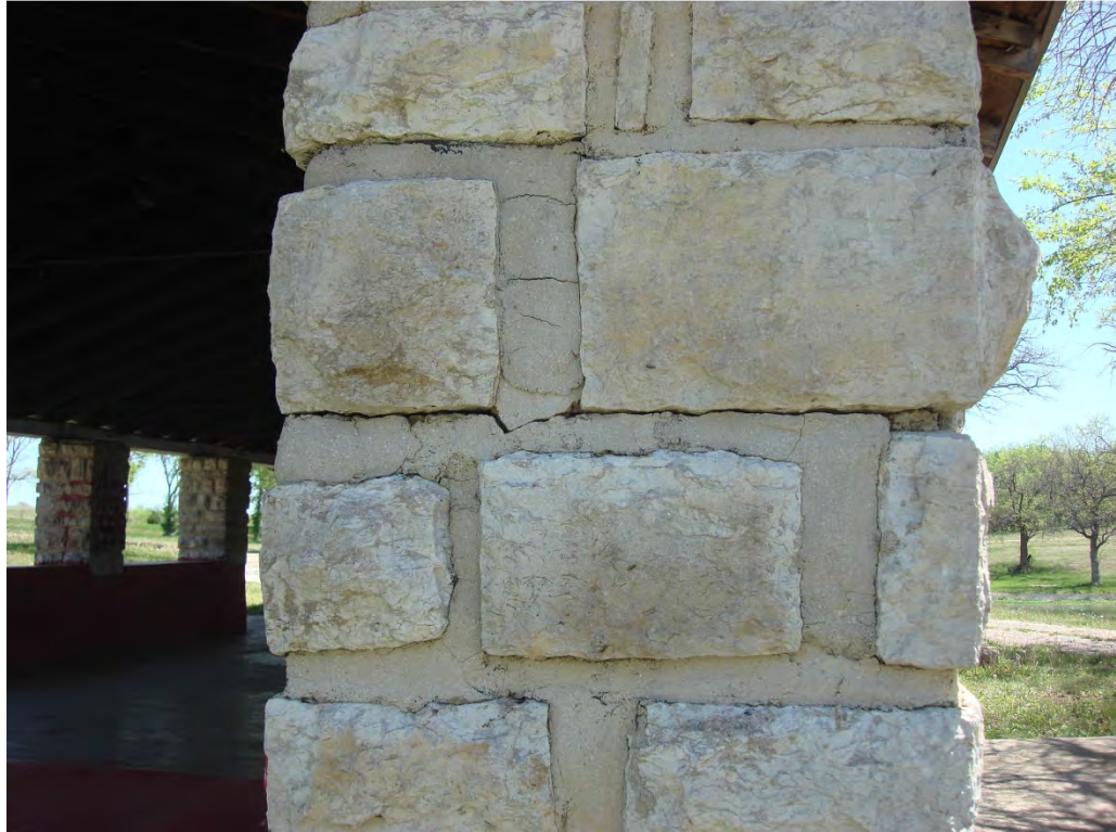
Typical horizontal crack along mortar lines in piers
