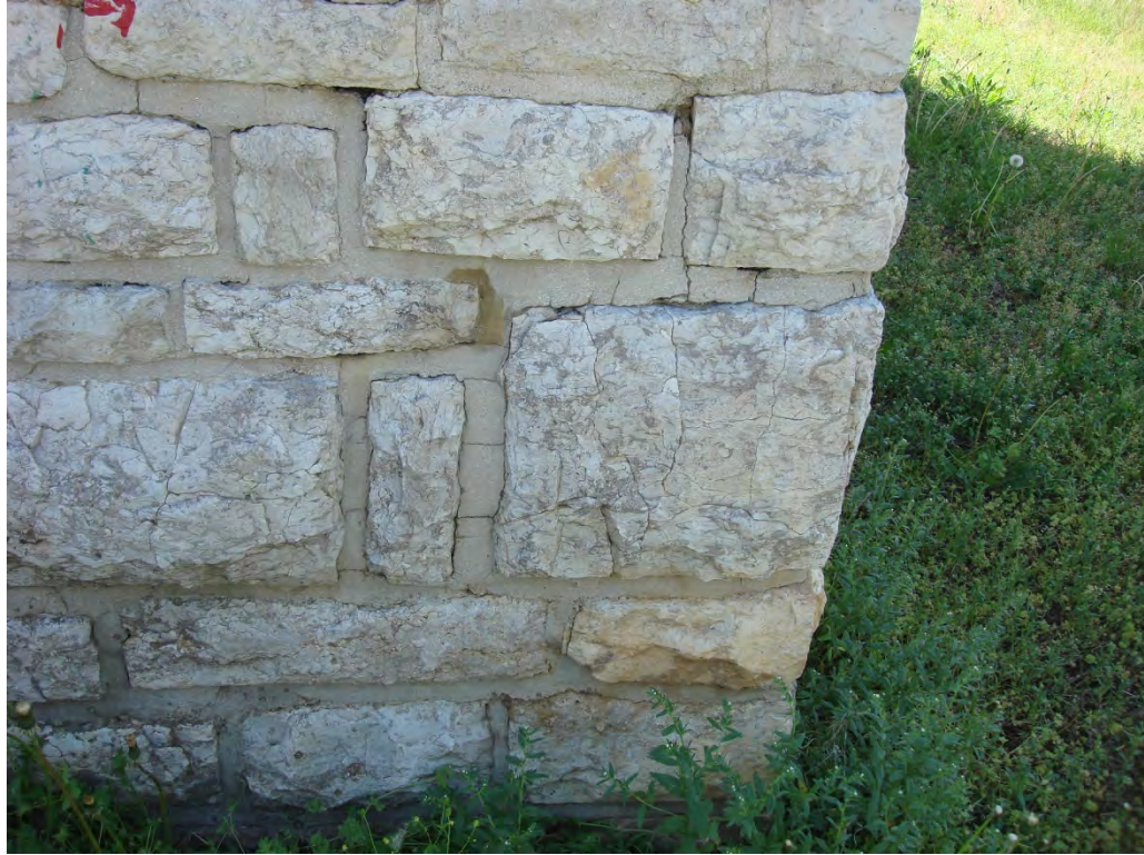
Moderate stress cracks in limestone blocks
