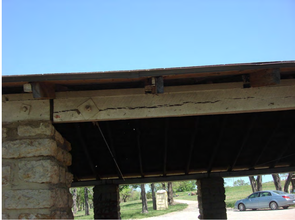
Typical horizontal cracks in timber beams supporting the roof structure
