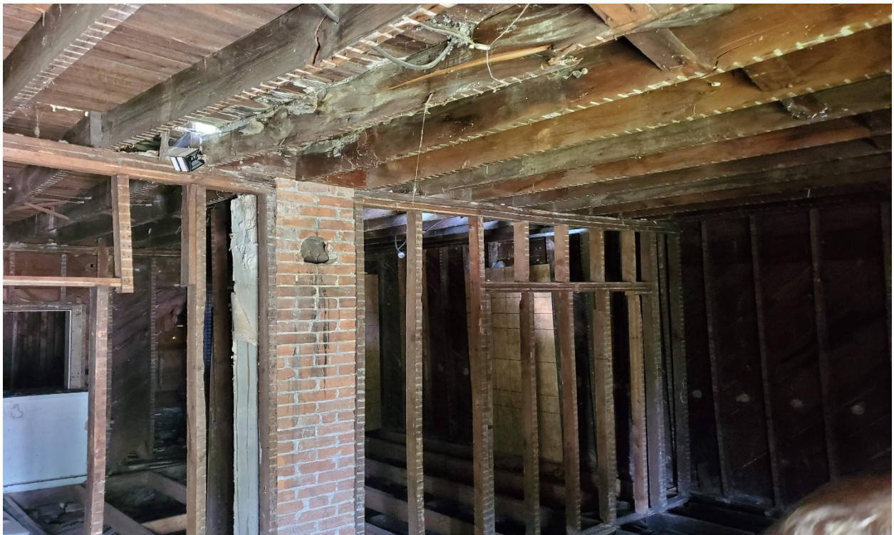
2 nd floor, floor joists cracked and broken
