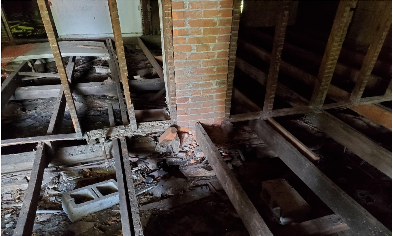
Chimney cracking, floor joists with little or no support with a load bearing wall sitting on them.
