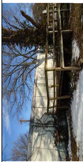
Front deck with a tree growing through the floor.
