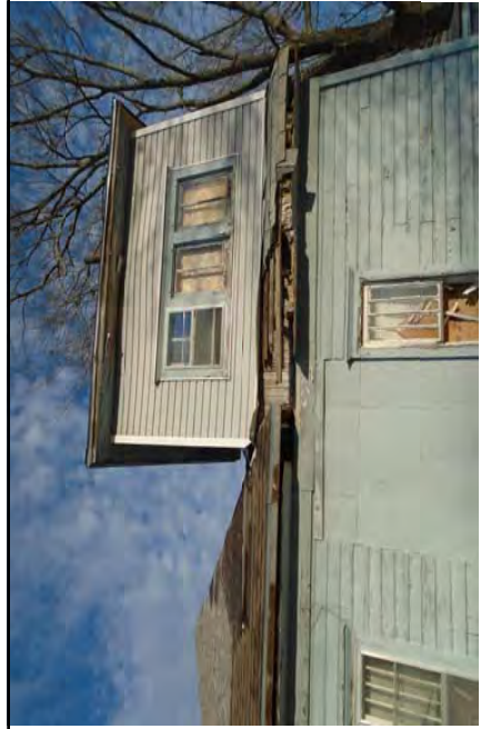
West side view showing the damaged roof, broken windows.
