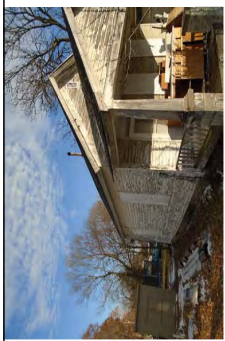
Side of house showing plastic over windows, the leaning front porch pillars
