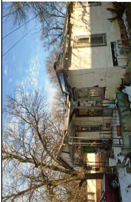
Front look at the collapsed roof
