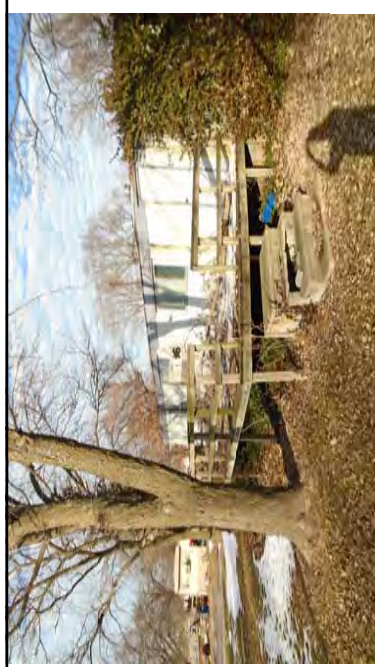
Front Yard showing the dangerous deck and shrubs growing up the side of the house.
