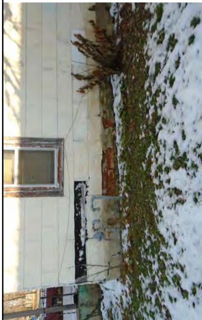
No gas meter, and falling foundation
